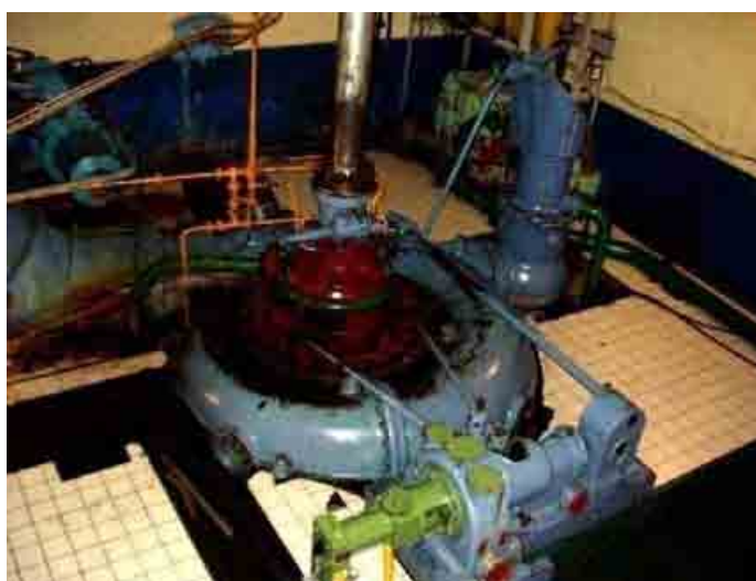
(b) Hydro Turbine
