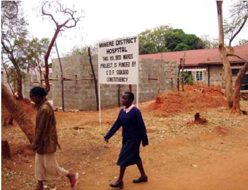
Ongoing construction for hospital ward financed by CDF; meanwhile Mbeere Hospital (located next right) lacked the most basic recurrent financing.
