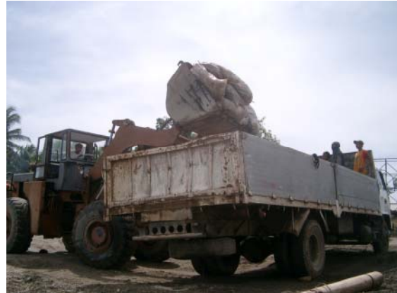
Loading Residual Waste to Dump Truck to Transport to the Proposed SLF (June, 2007)
