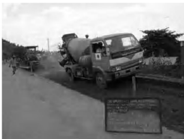
Date : 10/1/2008 ~ 11/1/2008 Activity : RN7 Base Course CRS Mixing and Leveling and Compaction Sta.1+500 ~ 1+660(EP) Right Side
