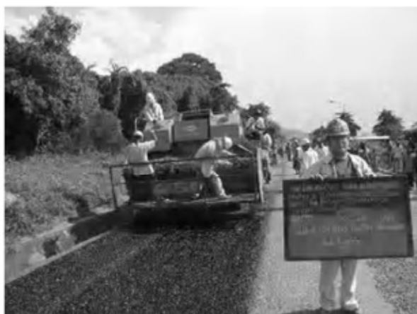
Date : 4/1/2008 ~ 16/1/2008 Activity : RN7 Double Bituminous Surface Treatment Prime Coat Sta.0+220~0+300 , 1+480~1+660(EP) Left 1st Layer Sta.0+220~0+300 , 1+480~1+660(EP) Left 2nd Layer Sta.-0+025~1+660(EP) Left
