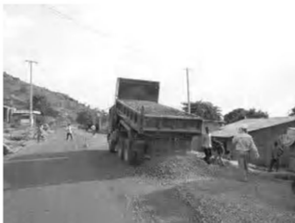
Date : 9/1/2008 Activity : RN7 Base Course CRS Dumping and Spreading Sta.1+500 ~ 1+660(EP) Right Side
