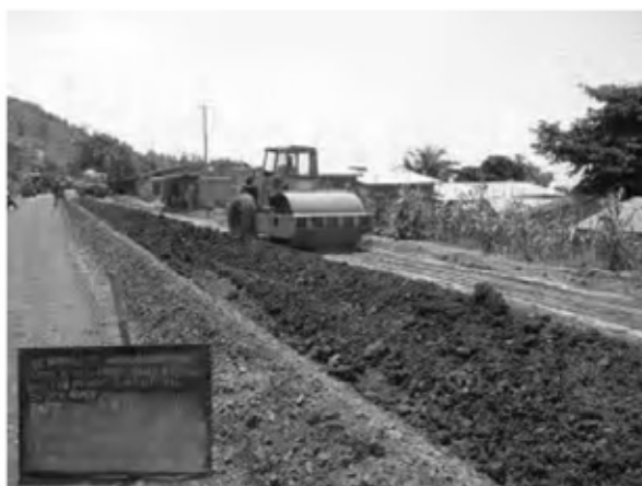
Date : 8/1/2008 ~ 9/1/2008 Activity : RN7 Sub-base Scarification and Back Filling Sta.1+500 ~ 1+660(EP) Right Side
