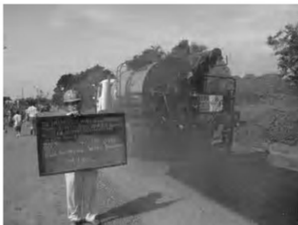
Date : 4/1/2008 ~ 16/1/2008 Activity : RN7 Double Bituminous Surface Treatment Prime Coat Sta.0+220~0+300 , 1+480~1+660(EP) Left 1st Layer Sta.0+220~0+300 , 1+480~1+660(EP) Left 2nd Layer Sta.-0+025~1+660(EP) Left
