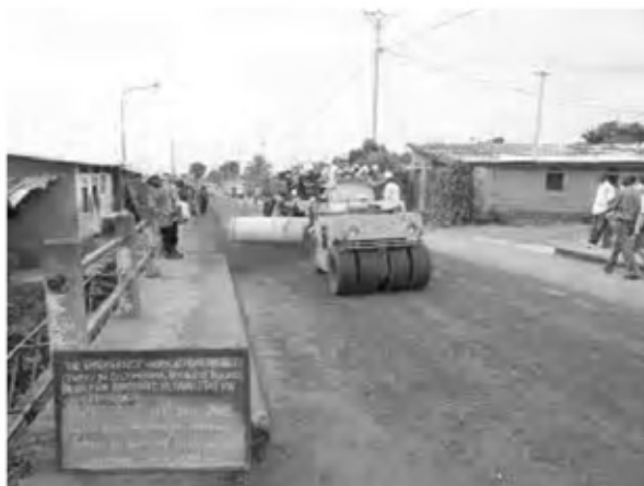
Date : 30 , 31/1/2008 Activity : RN7 Double Bituminous Surface Treatment Sweeping the Surface of Base Course Sta.-0+025~1+060 Right Side
