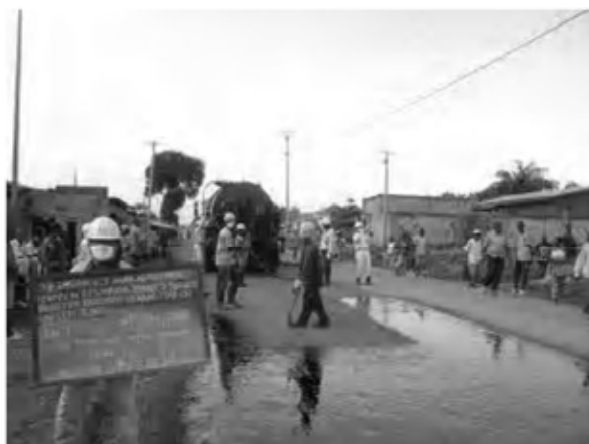
Date : 30 , 31/1/2008 Activity : RN7 Double Bituminous Surface Treatment Prime Coat Sta.-0+025~1+060 Right Side
