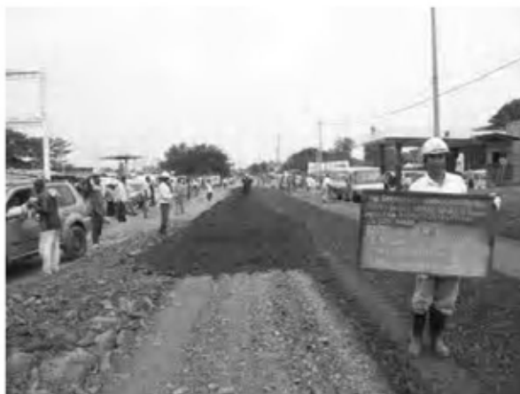
Date : 7/1/2008 ~ 8/1/2008 Activity : RN7 Sub-base Scarification and Back Filling Sta.1+500 ~ 1+660(EP) Right Side
