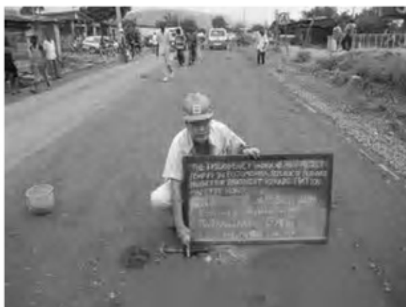
Date : 26 , 29 , 31/1/2008 Activity : RN7 Base Course Quality Control Thickness Check Sta.-0+025 ~ 1+060 Right Side
