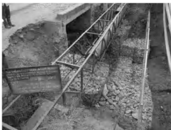
Date : 3/12/2007 ~ 12/12/2007 Activity : RN7 Protection for Erosion Gabion Mat Installation Sta.0+250 Bridge Lower Side
