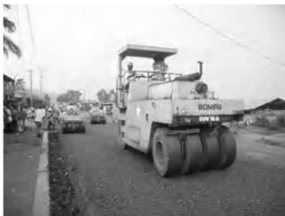
Date : 27/12/2007 , 28/12/2007 , 30/12/2007 Activity : RN7 Double Bituminous Surface Treatment 1st Layer Rolling Compaction Sta. -0+025 ~ 0+240 Left Side Sta. 0+280 ~ 1+500 Left Side
