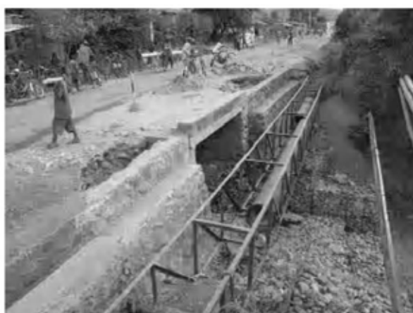
Date : 13/12/2007 ~ 21/12/2007 Activity : RN7 Protection for Erosion Stone Pitching and Rip Rap Back Fill and Compaction Sta.0+250 Bridge Lower Side
