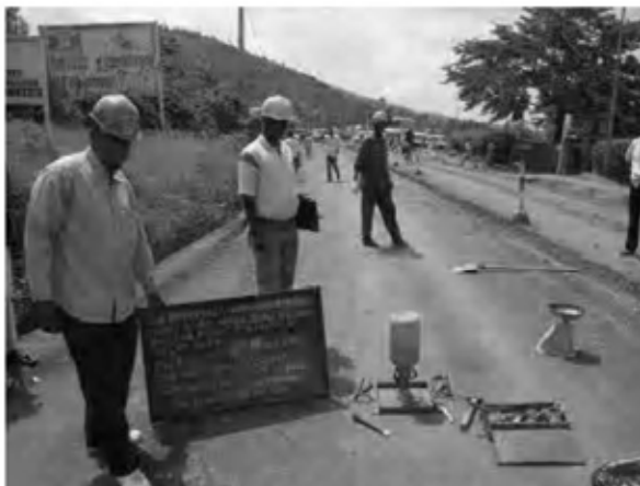
Date : 5/12/2007 , 28/12/2007 Activity : RN7 Sub-base Quality Control Field Density Test Sta.0+240~0+280 Left Side Sta.1+000~1+660(EP) Left Side
