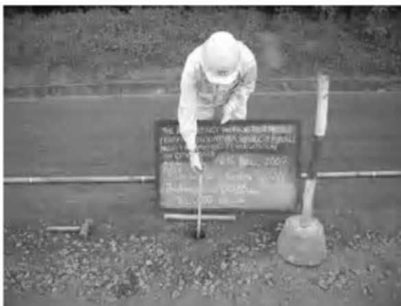
Date : 14/11/2007 ~ 30/11/2007 Activity : RN7 Base Course Quality Control Thickness Inspection Sta. -0+025 ~ 0+240 Left Side Sta. 0+280 ~ 1+500 Left Side
