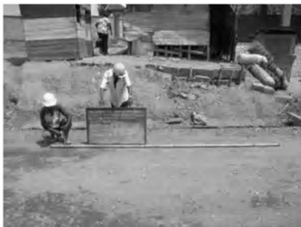
Date : 9/1/2008 Activity : RN7 Base Course Quality Control Smoothness Check Sta.1+500~1+660(EP) Left Side
