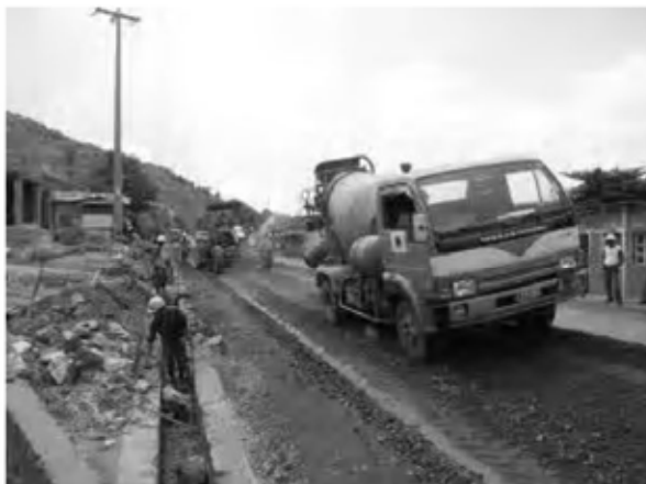
Date : 3/1/2008 ~ 6/1/2008 Activity : RN7 Base Course CRS Mixing and Leveling and Compaction Sta.1+500~1+660(EP) Left Side
