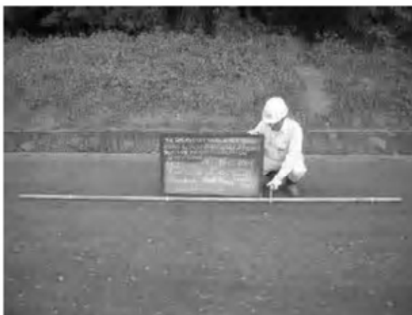
Date : 10/12/2007, 18/12/2007, 19/12/2007 Activity : RN7 Base Course Quality Control Smoothness Inspection Sta. -0+025 ~ 0+240 Left Side Sta. 0+280 ~ 1+500 Left Side
