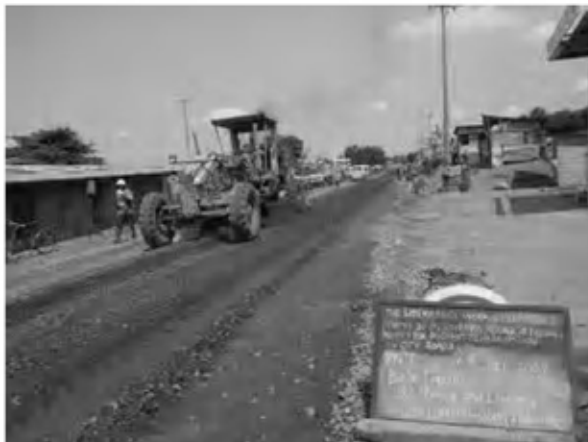
Date : 3/1/2008 ~ 6/1/2008 Activity : RN7 Base Course CRS Mixing and Leveling and Compaction Sta.1+500~1+660(EP) Left Side
