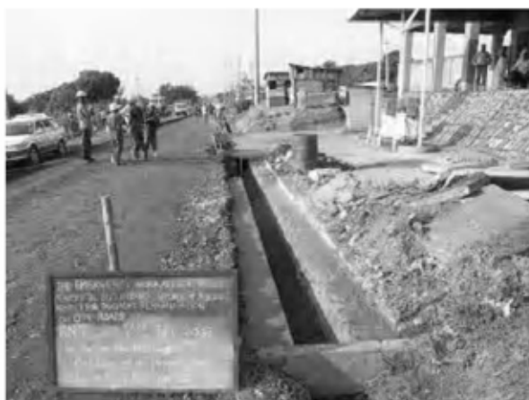
Date : 5/1/2008 ~ 9/1/2008 Activity : RN7 Repairing the Drainage Sta.1+600~1+620 Left Side Junction Sta.1+640~1+660 Entrance of the Fuel Station
