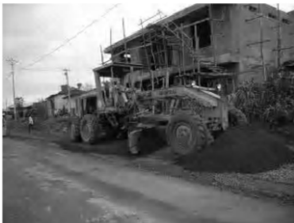
Date : 2/12/2007 ~ 14/12/2007 Activity : RN7 Base Course CRS and Powder Spreading Sta.0+540~1+500 Left Side
