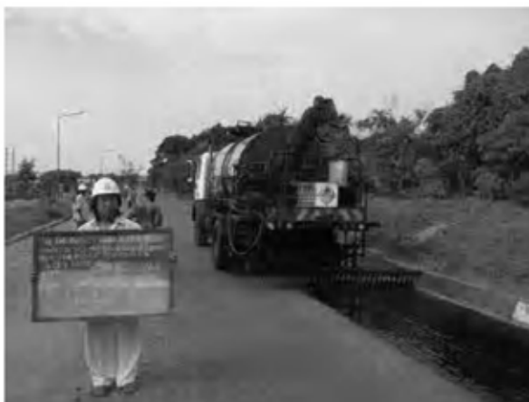
Date : 20 , 21 , 26 , 29/12/2007 Activity : RN7 Double Bituminous Surface Treatment Prime Coat Spraying the Primer Sta. -0+025 ~ 0+240 Left Side Sta. 0+280 ~ 1+500 Left Side
