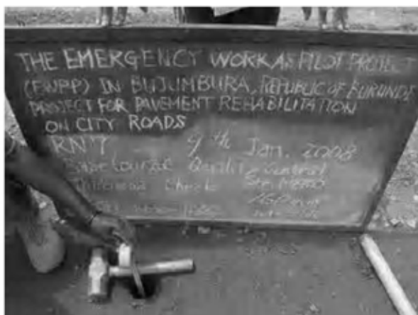
Date : 9/1/2008 Activity : RN7 Base Course Quality Control Thickness Check Sta.1+500~1+660(EP) Left Side
