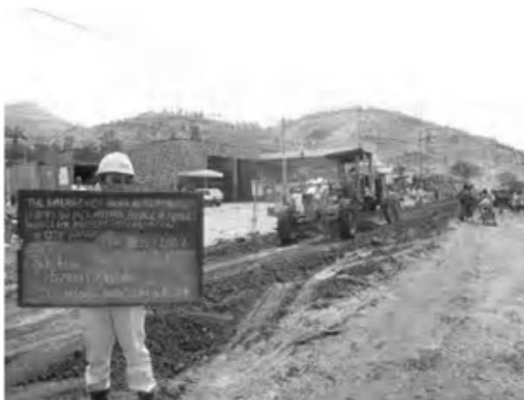
Date : 19/12/2007 ~ 26/12/2007 Activity : RN7 Sub-base Scarification and Compaction Sta.0+240~0+280 Left Side Sta.1+500~1+660(EP) Left Side & Right Side
