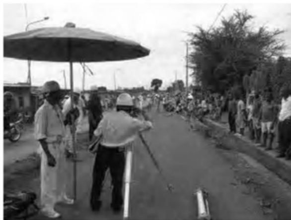
Date : 14/11/2007 ~ 30/11/2007 Activity : RN7 Sub-base Survey for the Finishing Level of Sub-base Sta. -0+025 ~ 0+240 Left Side Sta. 0+280 ~ 1+500 Left Side
