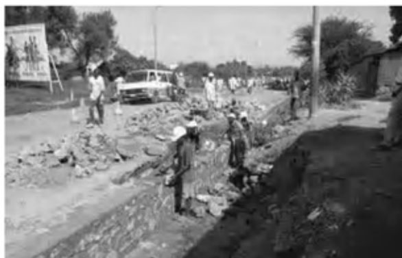
Date : 6/10/2007 ~ 31/10/2007 Activity : RN7 Protection and New Installation of Eroded Drainage Sta.0+200 ~ 1+500 Left Side
