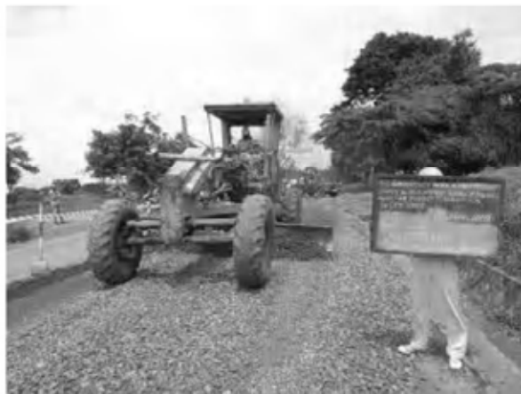
Date : 30/11/2007 Activity : RN7 Base Course CRS Mixing and Spreading Sta. -0+025 ~ 0+240 Left Side
