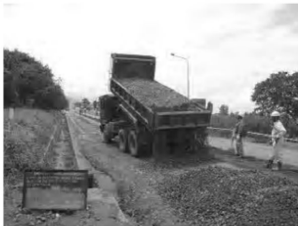
Date : 25/11/2007 ~ 30/11/2007 Activity : RN7 Base Course CRS Transportation and Dumping Sta. -0+025 ~ 0+240 Left Side Sta. 0+280 ~ 0+500 Left Side
