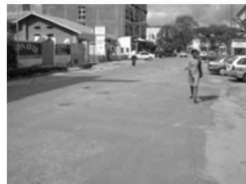
Evenness of pavement surface was not maintained ,that created pothole
