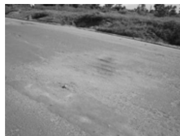
Pavement condition around starting point (Pothole was filled by unsuitable articles)
