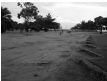
Parking spaces next to carriageway were provided but they does not look good condition
