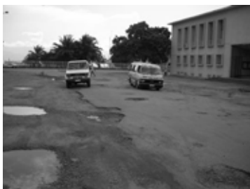
Many Potholes on entire road
