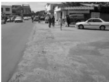
Provided pothole patching (not in good condition) at stating point of the road
