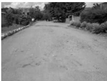
No tarmac pavement existed
