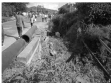
Heavy eroded road shoulder at No.2 +40 (near by cross box culvert)
