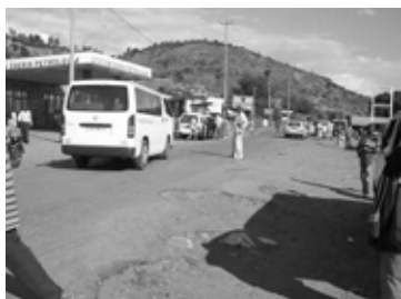
Deteriorated shoulder at No.15+40
