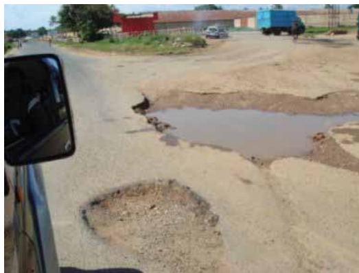
Deteriorated Road Surface
