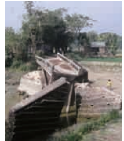
A concrete bridge that was damaged by flood during the rainy season
