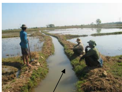
New watercourse constructed by farmers to get water up to tail portion
