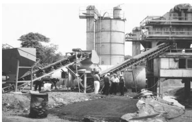
Asphalt Mixing Plat at Jabotabek Source: PT Saraya Karya
