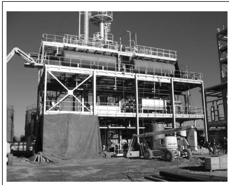
Figure A.1-8 View of BDF Plant (100 tpd)
