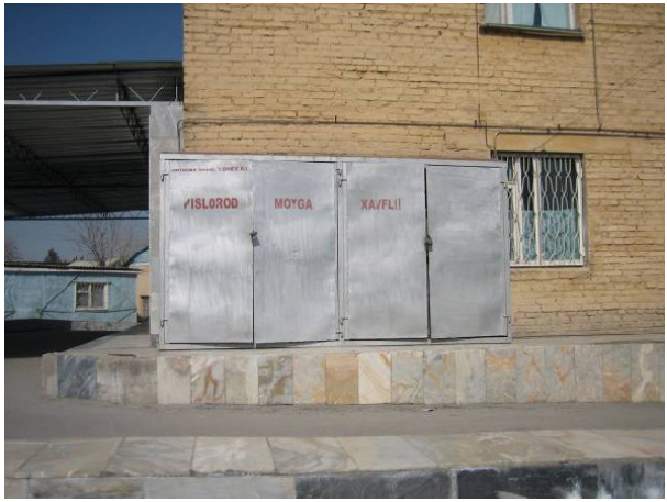
Oxygen manifold room for central gas supply
