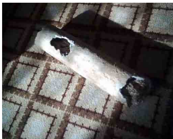
Damaged Asbestos Cement Pipe by penetration of Wooden Root
