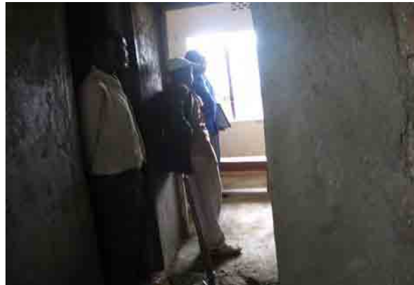
Management practice at Health Centers (HC) Construction of drug store with the support of community people
