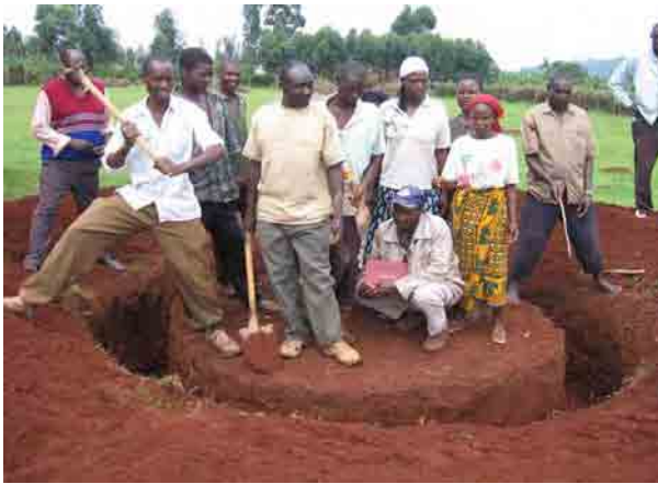
Maternity Care at Health Centers (HC) Excavation for water tank construction at Iranda HC with the support of community people
