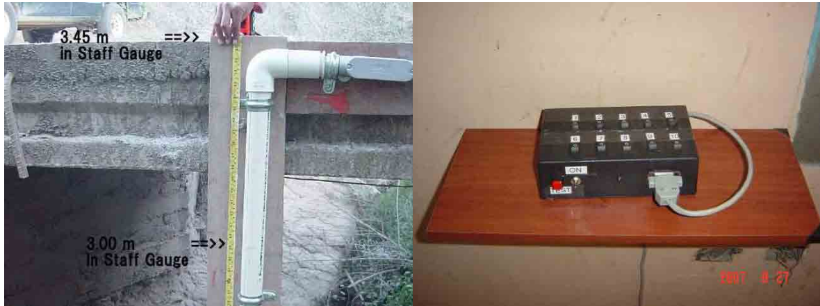
Photo S8-2-16 Comparison of the scale and Alarm box of Electrode type gauge
