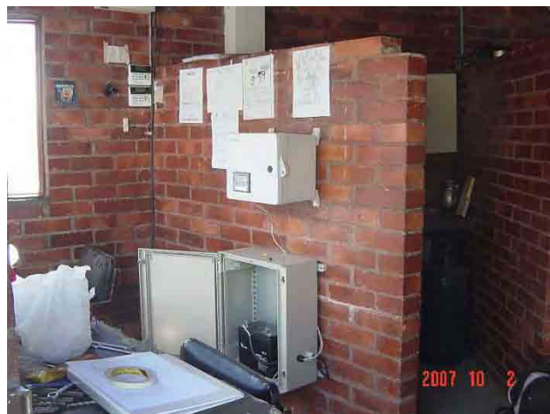
Photo S8-2-3 Data logger and Power supply in Moralba
