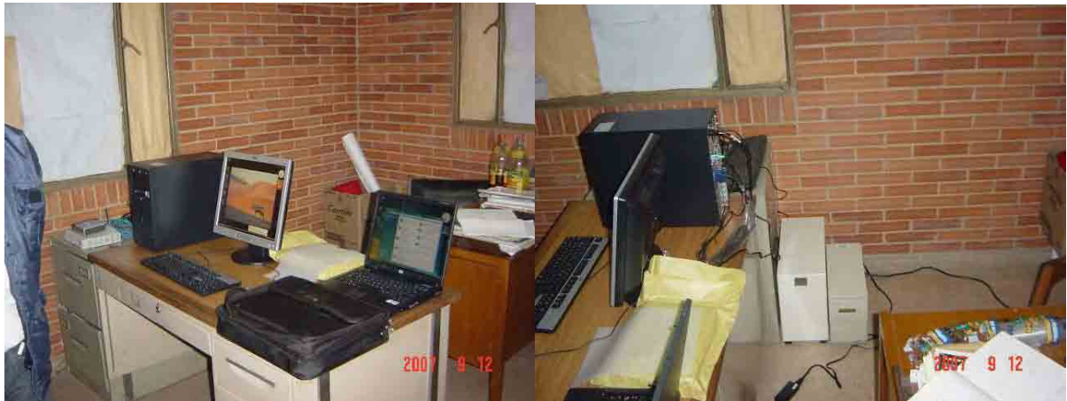
Photo S8-2-11 PCs, router and UPS in Firefighter Station
