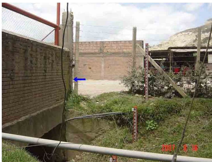
Photo S8-2-18 Water level of the flood in May 2006
