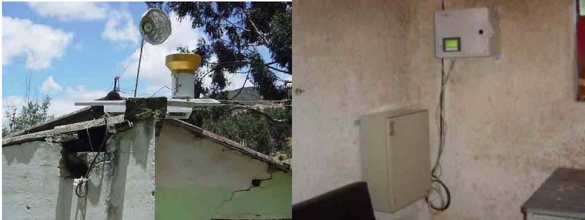
Photo S8-2-13 Rainfall gauge on the roof and Data logger and power unit
