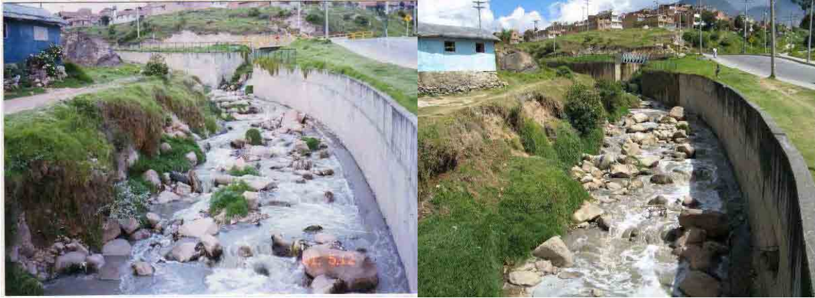
Photo S6-1-1 Riverbed Condition at Los Puentes in Chiguaza creek (Left: May 12, 2001, Right: January 16, 2007)
