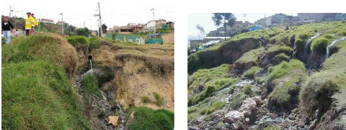
Photo S5-1-4 Water Flow into the Landslide
