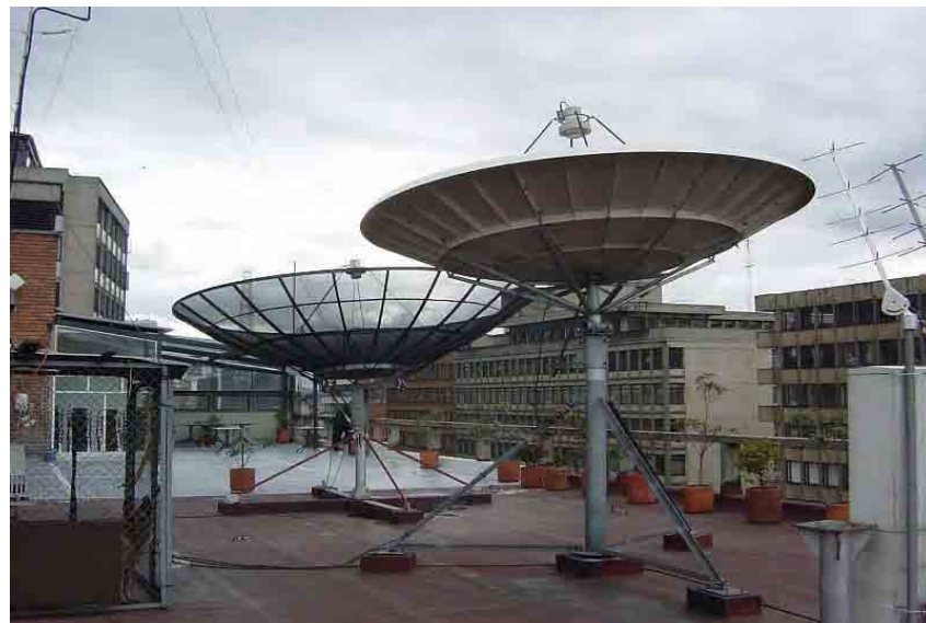
Figure S2-2-7 GOES Antennas on the Roof of IDEAM
