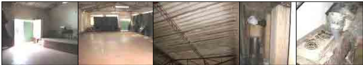
The Community Center at Florida I is an ample space, used during May 2006, which can hold up to 300 people. Nevertheless roof leaks, windows, ventilation and illumination, in bathroom and kitchen area is key. This center is owned by the neighborhood association. The Alcaldía CLOPAD coordinator explained that a legal procedure needs to be written promptly in order to make the required investments. Signing an agreement with the JAC board stating the center plays a shelter role in an emergency is one pending task to be achieved by the CLOPAD..
