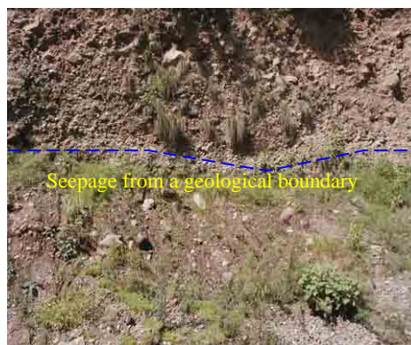
Figure 2.17 Seepage from the Geological Boundary (Source: JICA Study Team)
