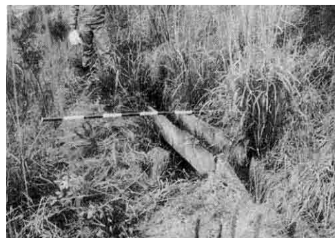
Figure 2.32 Water Leakages from a Joint of Drain and Erosion (Source: JH (1982), Slope Inspection Guide 1)
