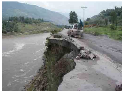
Figure 2.28 Embankment Failure caused by River Bank Erosion on Jhelum Valley Road (Source: JICA Study Team)
