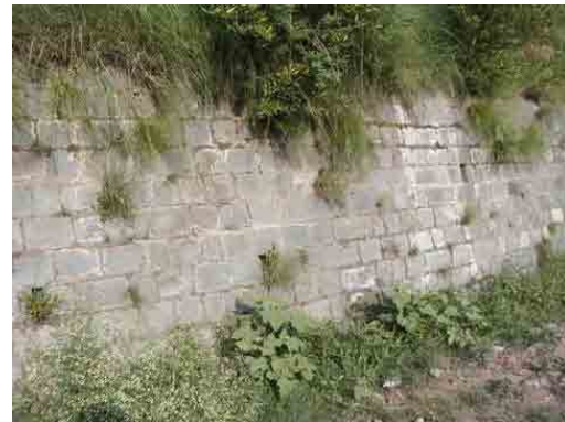
Figure 2.30 Grass Growing in Drain Pipes of the Retaining Wall (N-75) (Source: JICA Study Team)
