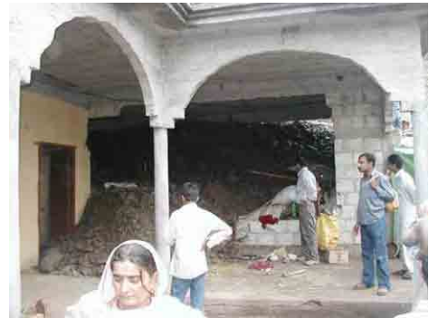
Figure 2.41 A Residential Building damaged by a Debris Flow, about 600 m long. Debris Flow deposits are composed mainly of Limestone Gravels of 10 cm-20 cm in diameter, (Source: JICA Study Team)
