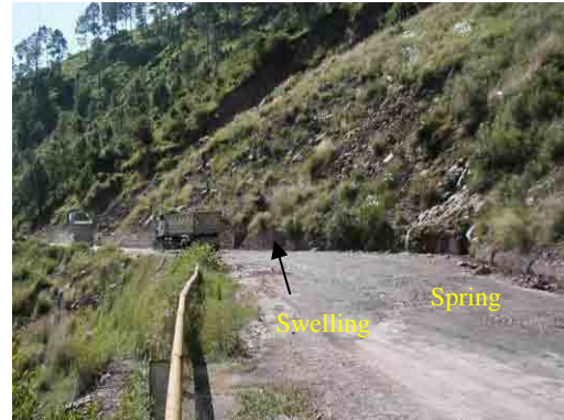
Figure 2.29 Swelling of Toe of slope on Jhelum Valley Road (Source: JICA Study Team)
