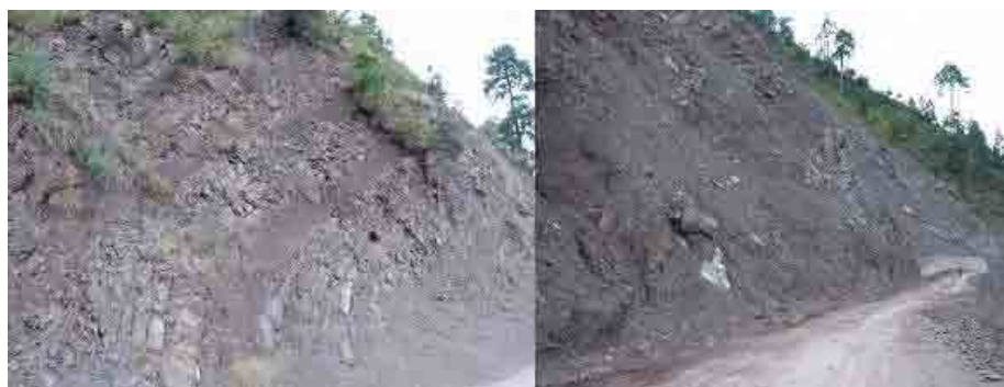
Photo 4.1.11 Typical flexural toppling and failure of alternating beds of sandstone and mudstone in Jaskool
