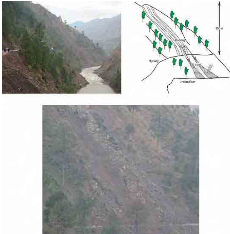
Figure 4.1.6 Slope failure with buckling of beds in the north of Jaskool: Buckled part 10 m above the road (upper right and lower photos).
