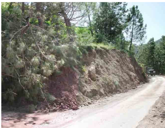
Photo 4.1.4 Active middle size landslide near Dhellan
