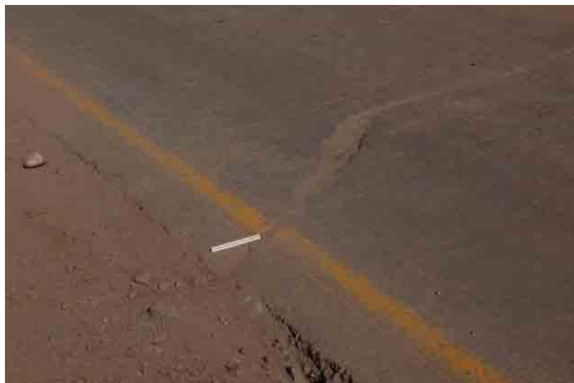
Photo.3.5.12 Slight displacement of road pavement as a sign of a deep active landslide
