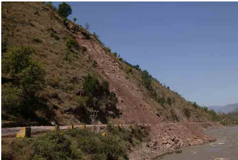
Photo 3.5.10 Reactivated landslide due to toe erosion
