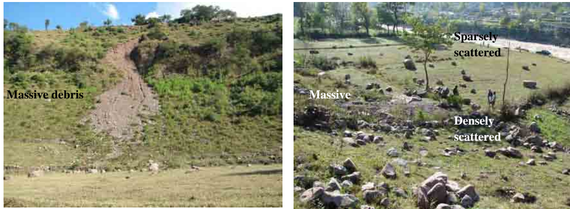
Figure 3.9.3 Slope failures on the terrace scarp of site 7.
