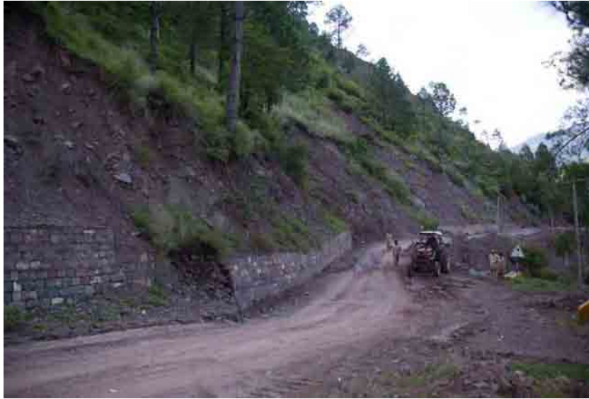
Photo.3.5.13 Dislocation of retaining wall due to active land-sliding of weathered rock or earth
