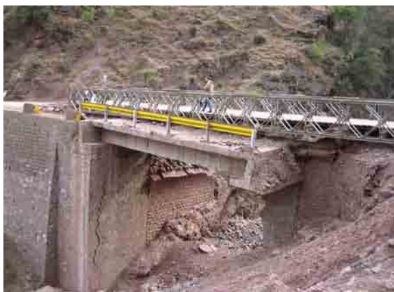
The old bridge damaged by the earthquake
