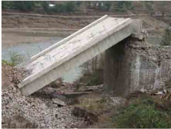
The old bridge damaged by the earthquake
