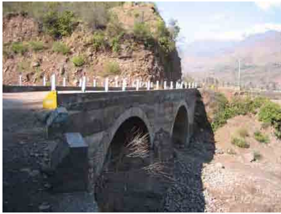
The old bridge damaged by the earthquake
