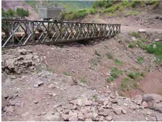
Old bridge damaged by the earthquake
