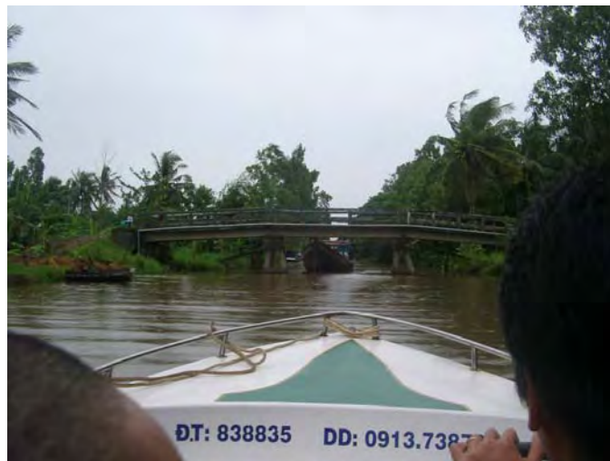
1.5 – 2.5 m clearance between the girders and the water level is required for navigation even for a small canal.
