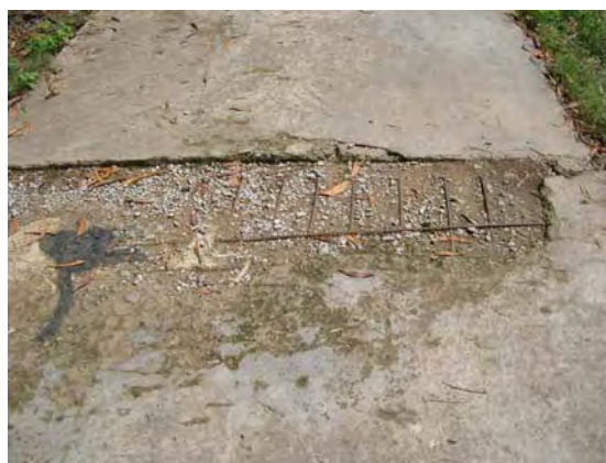
Deterioration of concrete road paving
