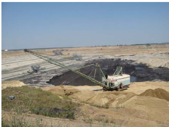
A main machine to strip waste in the Drmno Mine, Kostolac Mine is a dragline.
