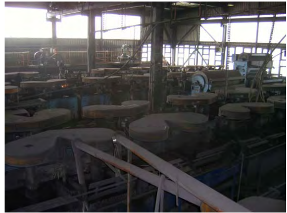
Flotation Stage at Rudnik Mine Processing Plant (2)
