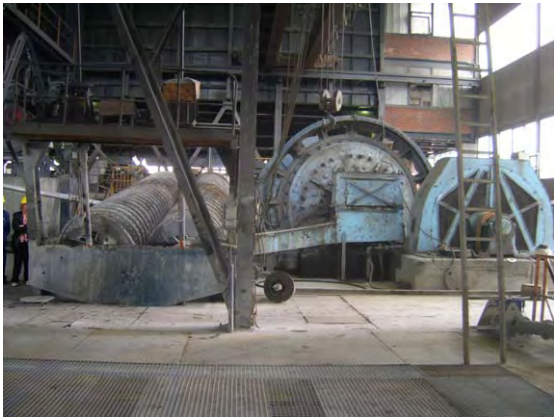
Grinding stage at Rudnik Mine Processing Plant
