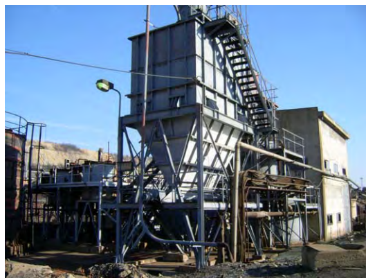
Waste water treatment plant
