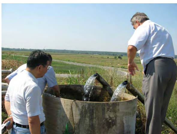
Around the Drmno Mine, there are about 200 wells which are continuously dewatering.
