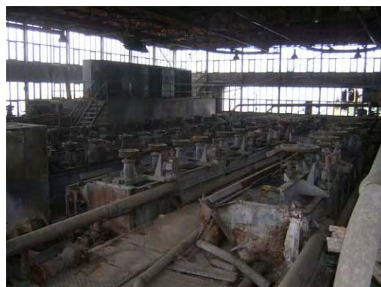
Flotation stage at Suba Ruda Mine Processing Plant
