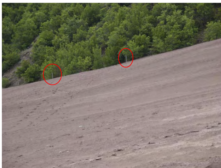
The Well to measure Water Level in the Dam Body
