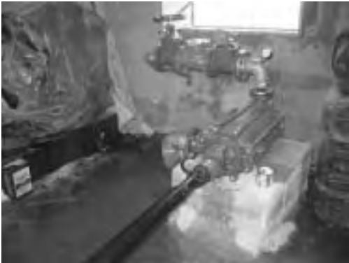
Installed Horizontal Pump and Accessories for Booster
