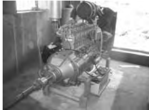
Installed Diesel Engine for Well
