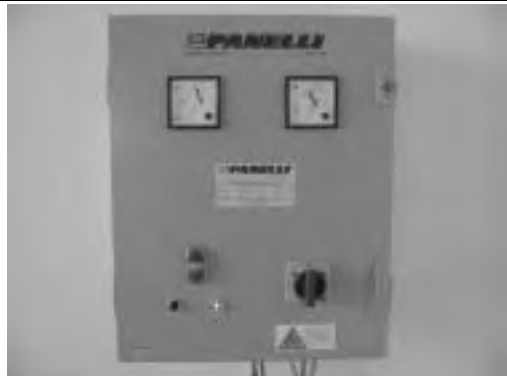
Control Panel for Pump
