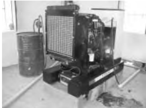
Diesel Engine Generator (45kVA)
