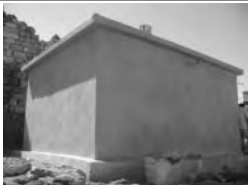
Existing Ground Water Tank (25m 3 ) constructed by GARWSP
