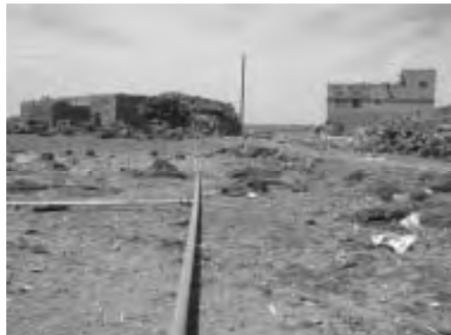
Installed Distribution Main
