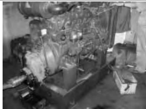
Diesel Engine for Booster before Replacement
