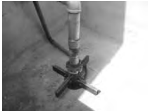
Inside Pump Pit (after Installation of Pump and Pipe)
