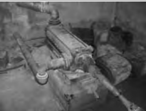
Horizontal Pump for Booster before Replacement
