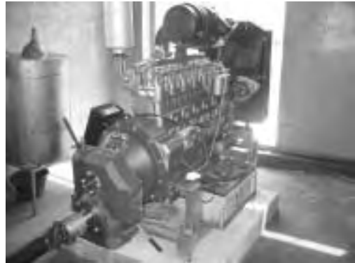
Installed Diesel Engine for Booster
