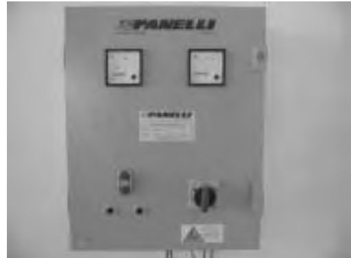
Control Panel for Pump
