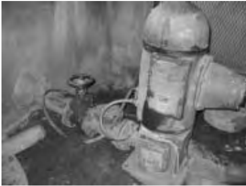
Vertical Shaft Pump for Well before Replacement
