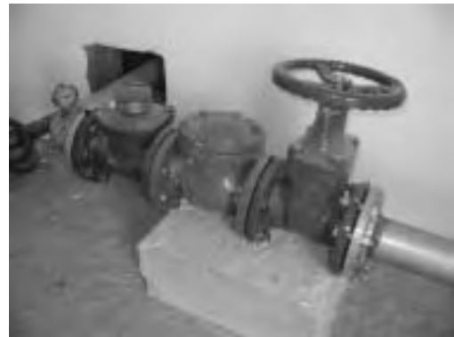
Accessories (Pressure Gauge, Water Meter, Check and Gate Valves)
