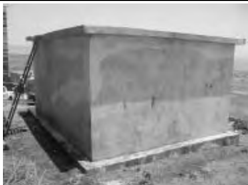
Water Leakage of Existing Ground Water Tank (25m 3 )
