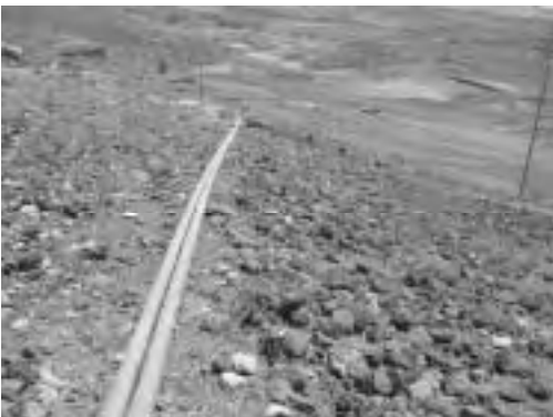
Installed Pumping and Distribution Main
