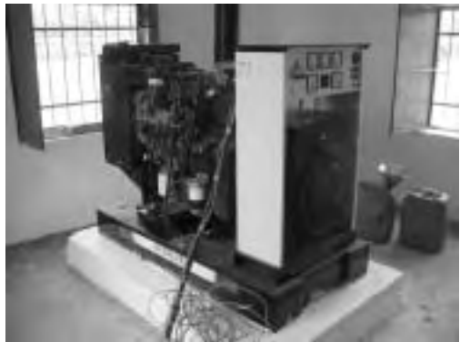
Diesel Engine Generator (45kVA)
