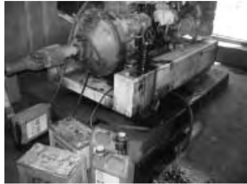
Diesel Engine for Well before Replacement
