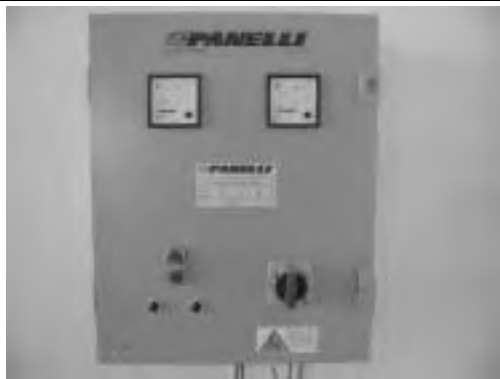
Pump Control Panel (Switch, On/Off Button, Meters)
