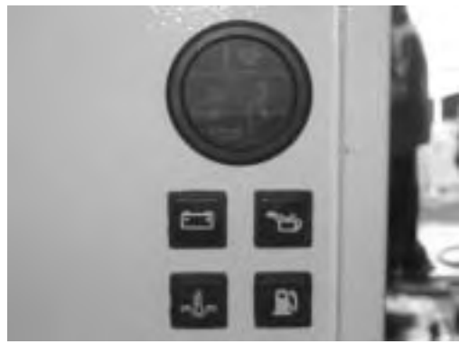
Generator Panel (Green & Red Lights and Indicators)
