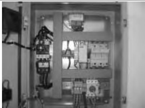
Inside Control Panel (do NOT touch)
