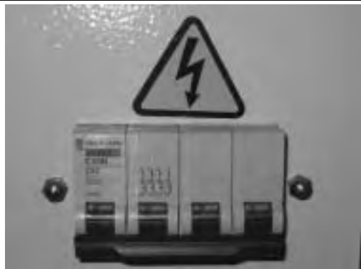
Circuit Breaker (Up - On, Down - Off)
