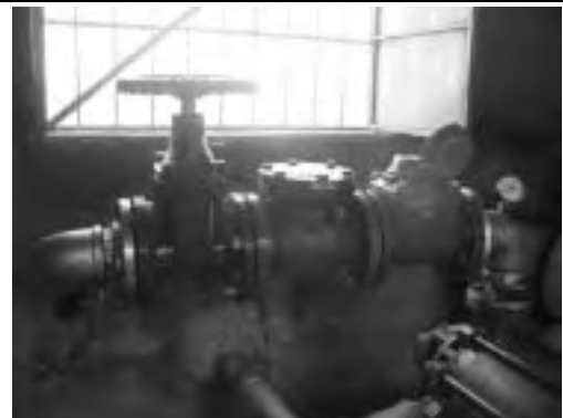
Accessories at Booster Pump House (from right: Pressure Gauge, Water Meter, Check Valve and Gate Valve)
