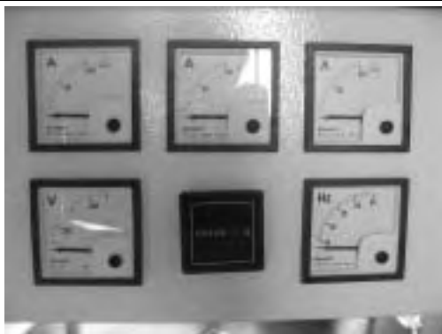
Generator Panel (Ampere, Voltage and Frequency Meters)
