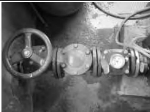
Accessories at Well Pump House (from right: Pressure Gauge, Water Meter, Check Valve and Gate Valve)
