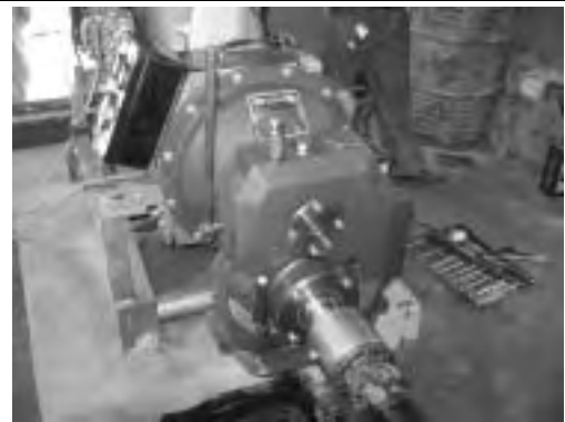
Gear Box and Lever for Cardan Shaft of Pump for Booster
