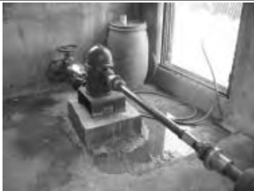
Cardan Shaft of Pump for Well
