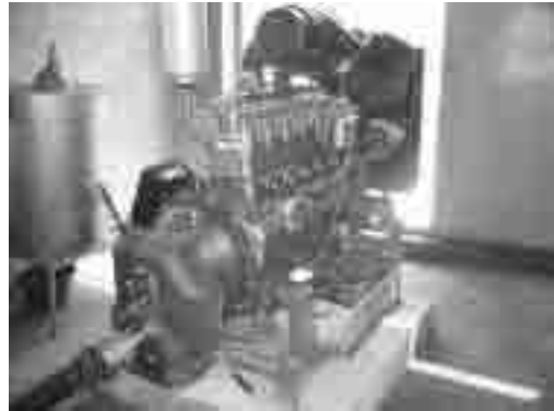
Installed Diesel Engine for Booster
