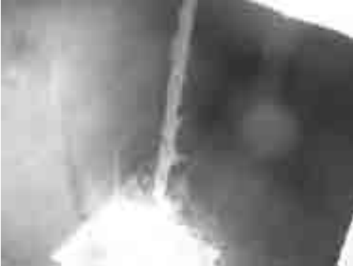
Water Flowing in Existing Ground Water Tank
