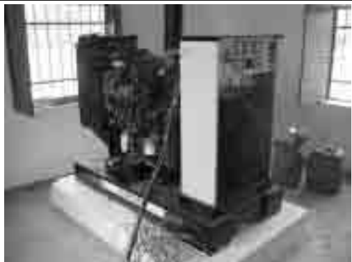
Diesel Engine Generator (45kVA)
