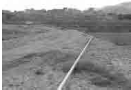
Installed Pumping Main (3")
