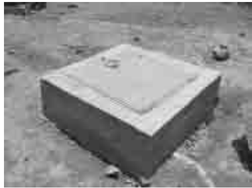
Valve Chamber along Distribution Main
