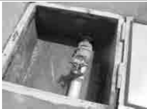
Gate Valve and Water Meter beside Fountain at Mosque
