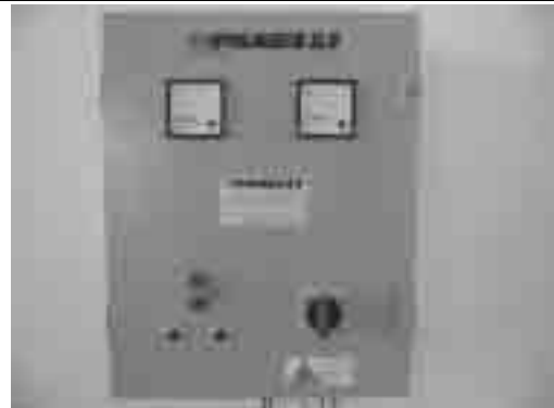
Control Panel for Pump
