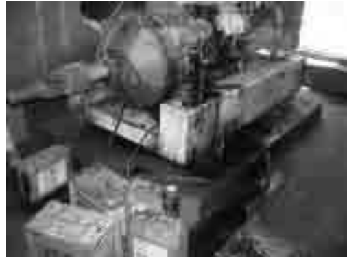
Diesel Engine for Well before Replacement
