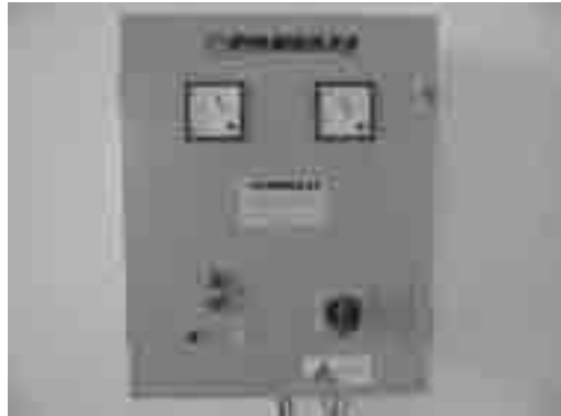
Control Panel for Pump
