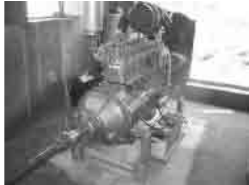
Installed Diesel Engine for Well
