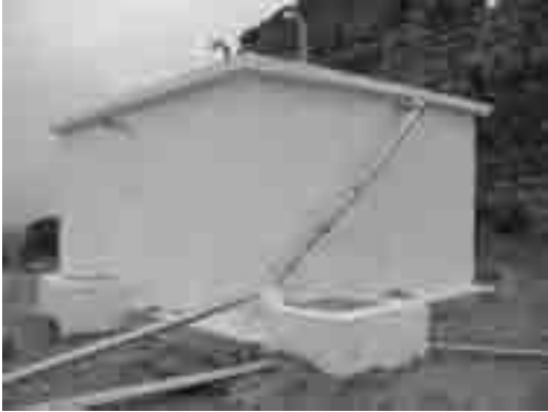
Rehabilitated Existing Ground Water Tank (25m 3 )
