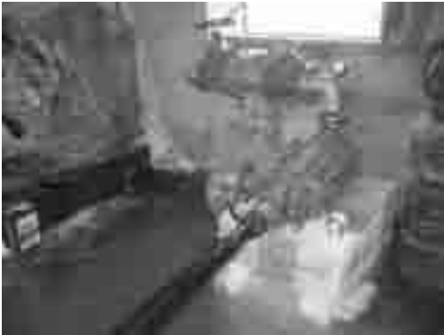
Installed Horizontal Pump and Accessories for Booster
