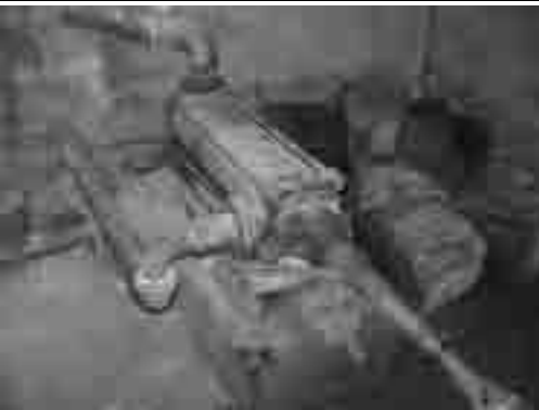
Horizontal Pump for Booster before Replacement
