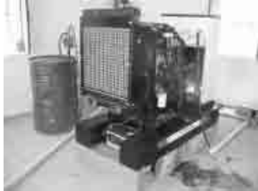
Diesel Engine Generator (45kVA)
