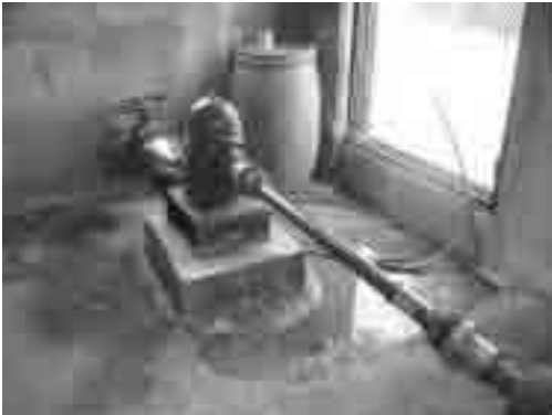
Installed Vertical Shaft Pump and Accessories for Well
