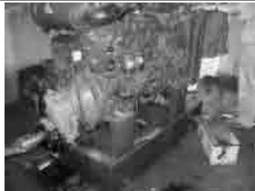
Diesel Engine for Booster before Replacement
