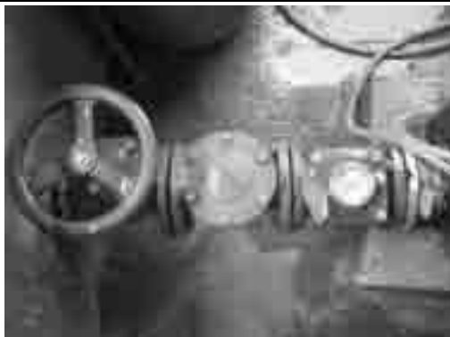
Accessories at Well Pump House (from right: Pressure Gauge, Water Meter, Check Valve and Gate Valve)
