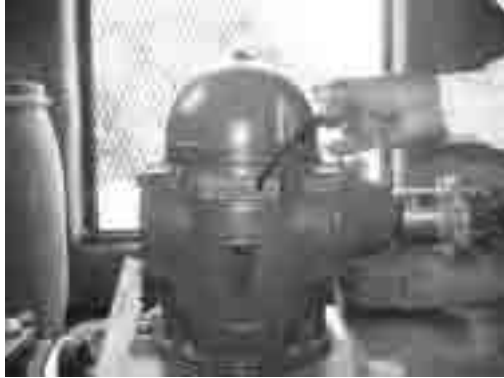
Lubricant Oil of Pump Drive Unit (Head) for Well
