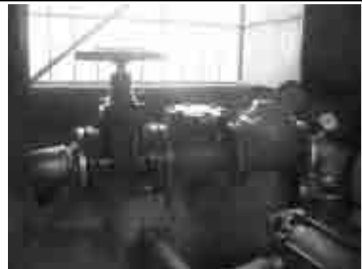
Accessories at Booster Pump House (from right: Pressure Gauge, Water Meter, Check Valve and Gate Valve)
