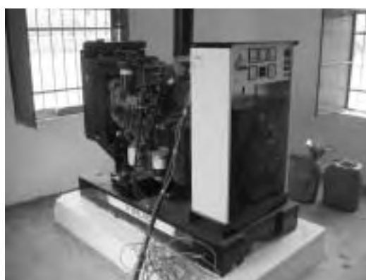
Installed Engine Generator
