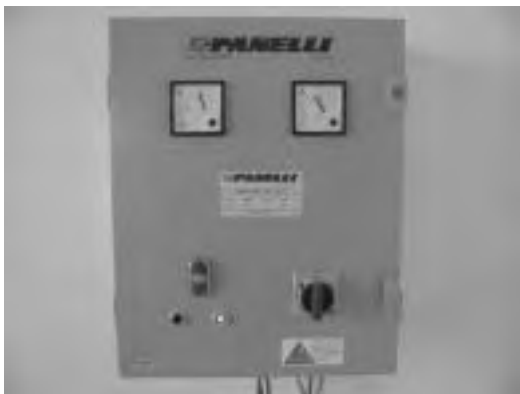
Installed Control Panel for Well Pump
