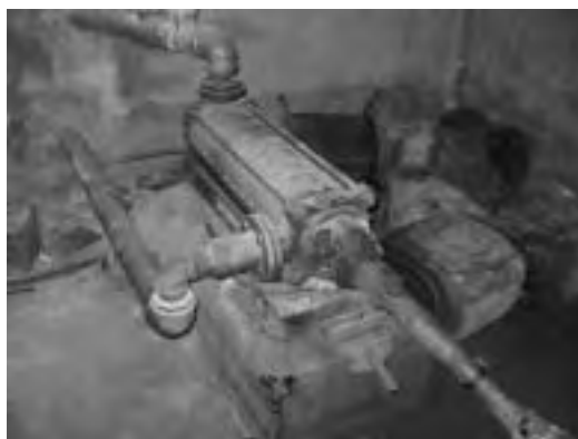
Booster Pump before Replacement
