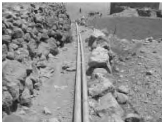
Pumping Main (left) and Distribution Main (right)
