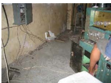
Arrangement of cables
