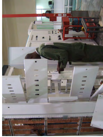
Electric Switch control Panel
