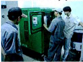
F.10 Installation and operation of electric generator
