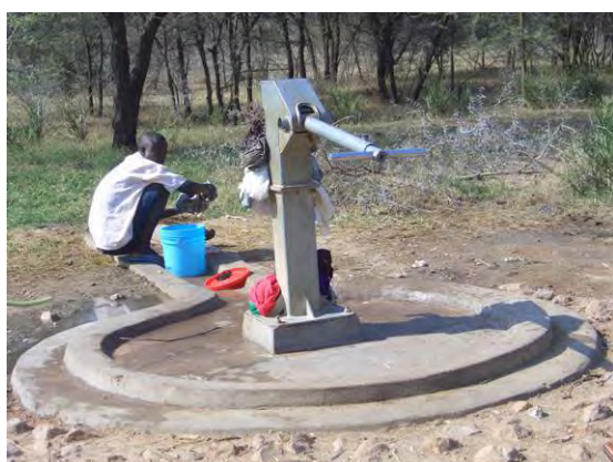
Gula - borehole used for washing only (24.9 mgF - /L)
