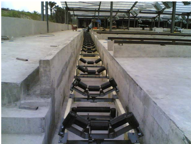
Photo 16: Conveyor Belt system being installed at the end of the drying beds for transfer to storage silos.
