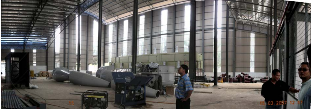
Photo 13: Interior of the FELDA Bkt Sagu OPF Plant. Equipment such as silos and blower are in the process of being installed.
