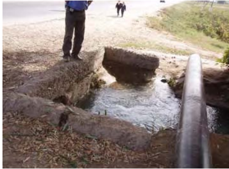
Inlet of a cross-drainage pipe flooded with drained irrigation water near the distance mark of 31 + 000 km
