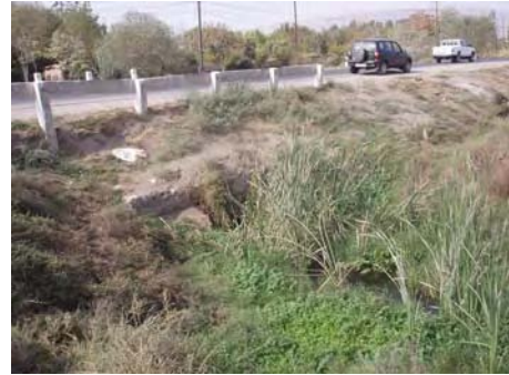
Inlet of a cross-drainage pipe filled with sediment near the distance mark of 30 + 000 km
