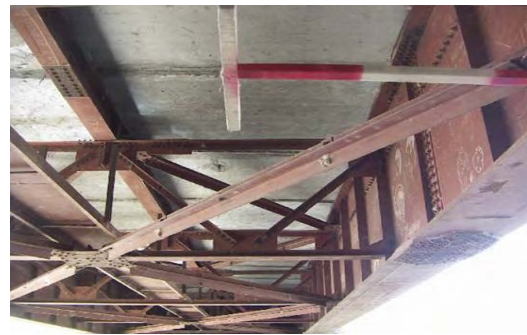
Fig. 2-8 State of Painting of the Super-Structure of Existing Bridge No. 7
