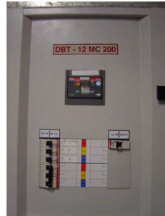
Switchboard installed at corridor
