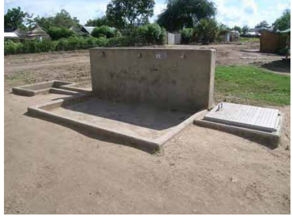
One of Hydrants
