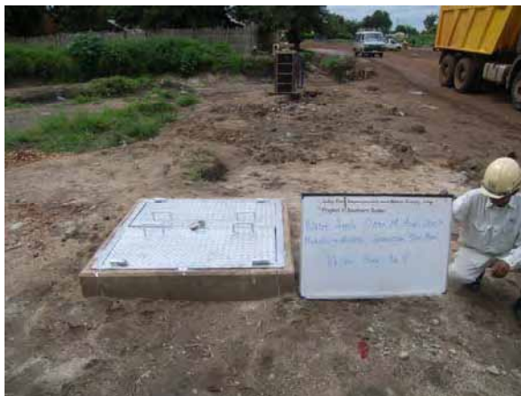
Valve Box at Connection Point with Existing Pipe Line
