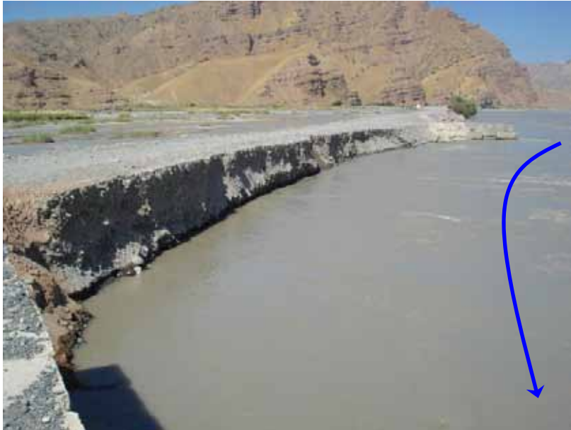
Fig. R 11.4.7 Damage of Spillway Guide Dike (around 1.0km )
