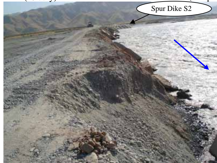
Fig. R 11.4.5 Damage of Main Dike 2 (From Downstream, 1 August)
