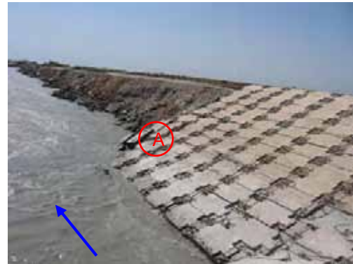
Fig. R 11.4.4 Damage of Main Dike 2 (1 September)
