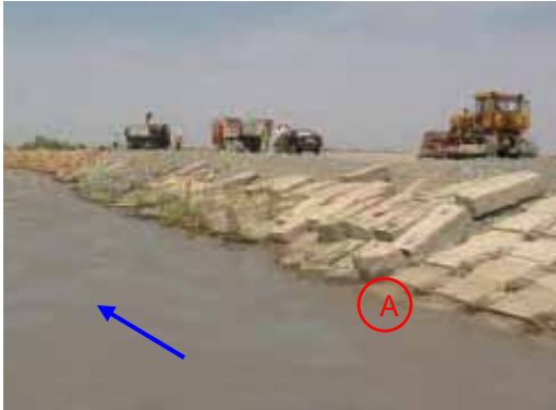
Fig. R 11.4.3 Damage of Main Dike 2 (25 July)
