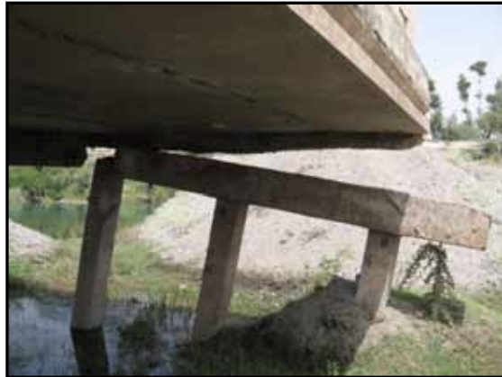
Damaged concrete piles
