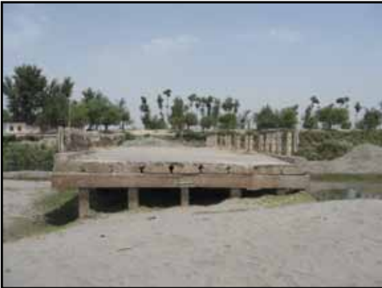
Sedimentation along the piles
