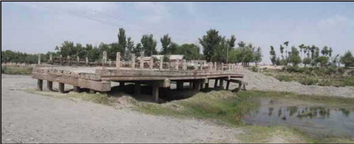
Size of the Bridge is 20.0 m long and 8.0 m wide. Four (4) spans with five (5) lines of five (5) concrete piles (350 mm x 300 mm). Length of concrete pile is 8.0 m (based on the site interview).
