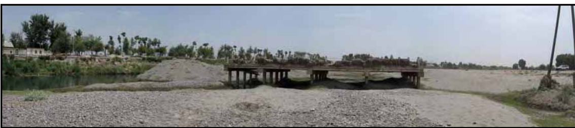
Waterway is changed after the flood and bridge is isolated in the middle of river
