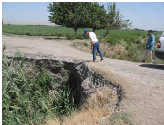
Fig. R 8.8.2 Asphalt Paved Pipe Culvert on the Evacuation Route #3 between Sovetobod and Iqbol in Jamoat Turdiev
