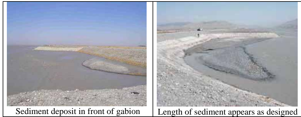
Fig. R.2.5.4 Sediment Deposits behind Spur-dike in Hamadoni District
