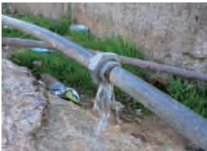
Water leaking from a drain
