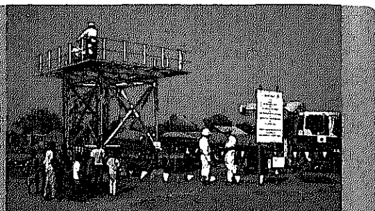
Construction site of a water supply facility: Development of basic infrastructure is urgently required in Sudan. (Emergency Study on the Planning and Support for Basic Physical and Social Infrastructure in Juba Town and the Surrounding Areas)
