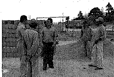
Construction site of a primary school, which is assisted by the project with the participation of the community
