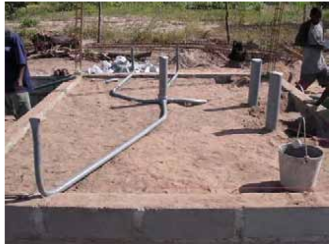
Sewage piping: Public Toilet Shed
