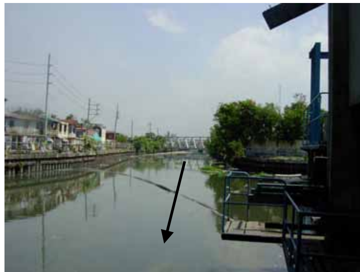
Inlet of Tripa de Gallina Drainage Pumping Station as of March 3, 2007
