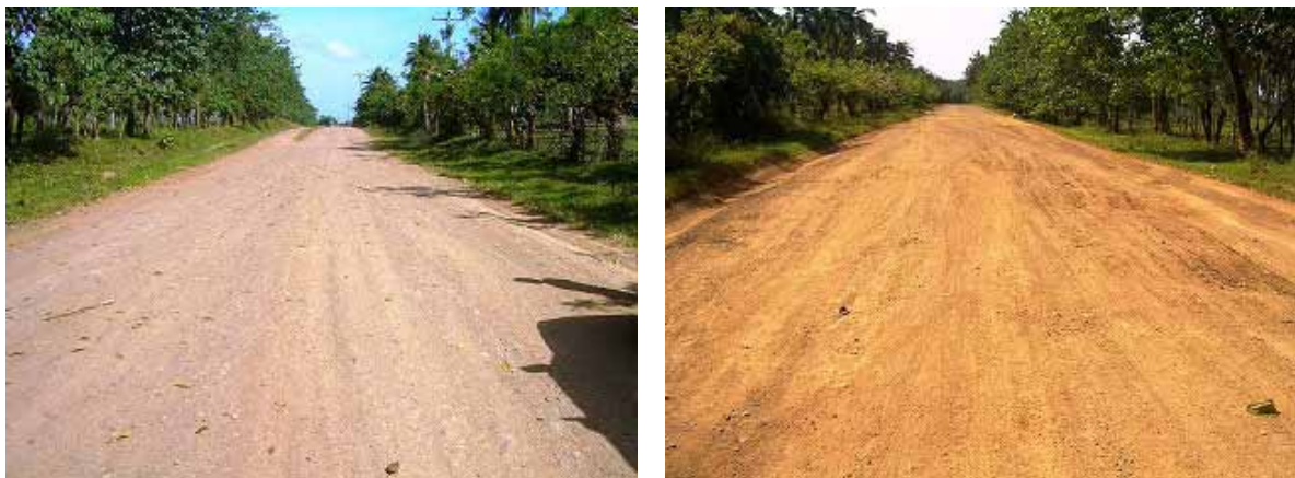
Figure 5-9 Existing Road Condition of Masbate – Aroroy Section
