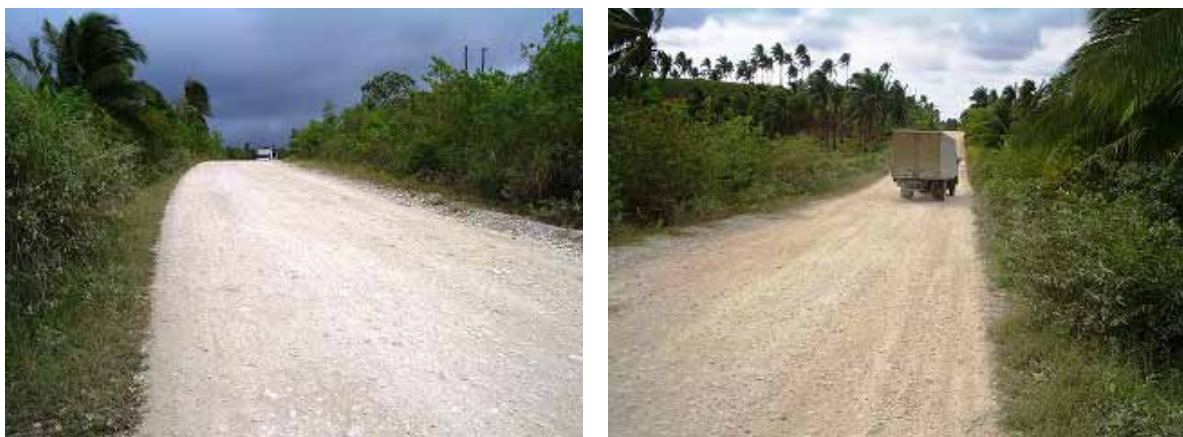
Figure 5-5 Existing Road Condition of Cataingan – Esperanza Section (municipality road)
