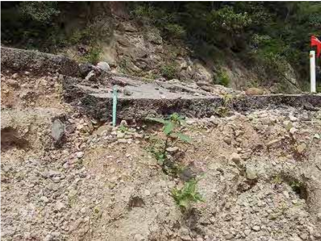
Photo 9.7.9 Depression in upper part of the landslide
