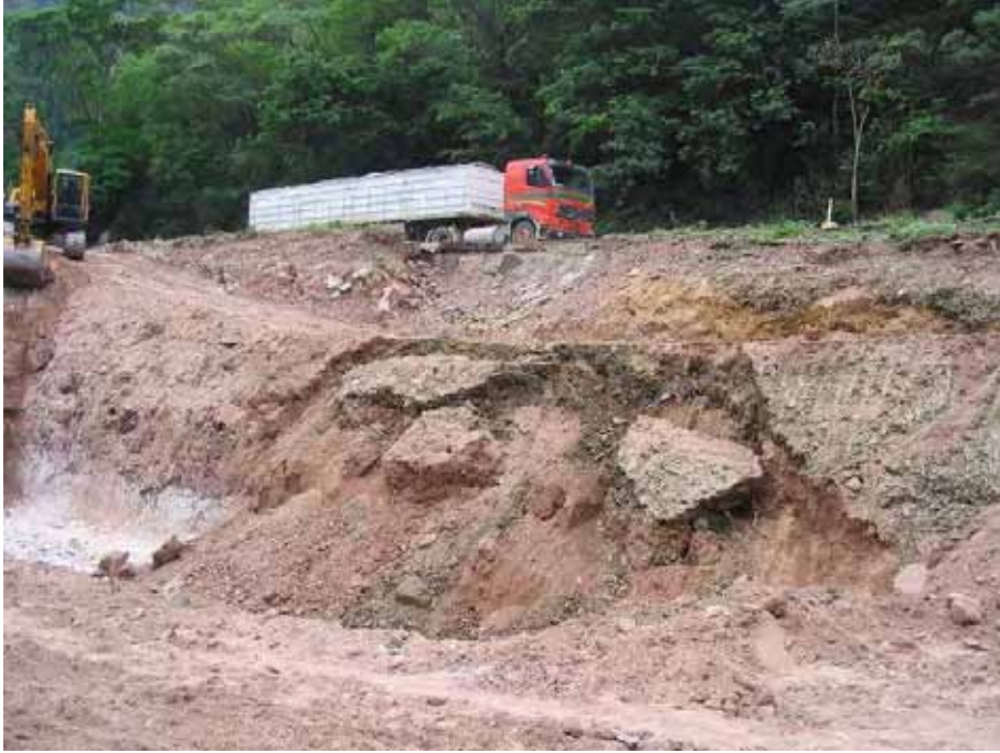
Photo 9.11.1 Slope failure due to the poor construction work of the original road body
