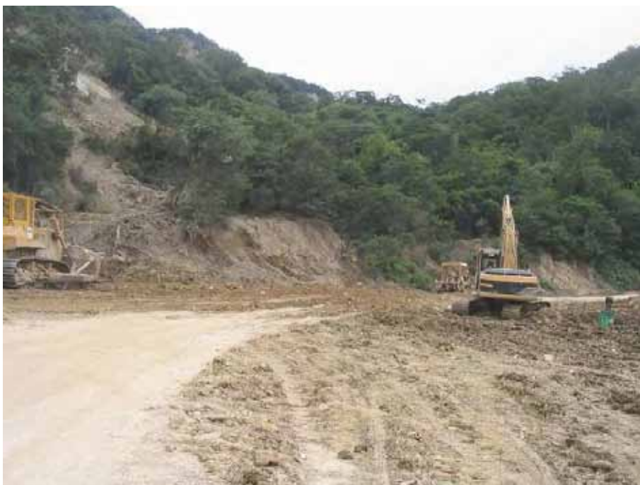
Photo 9.13.4 Collapsed road by debris flow (restoration work is under way)
