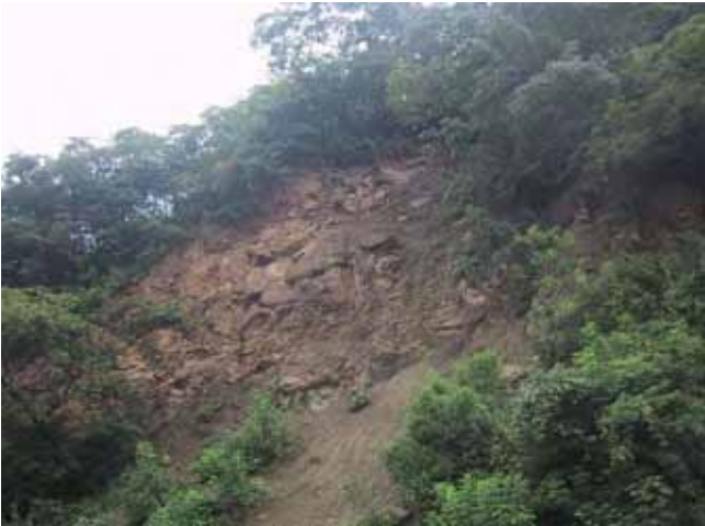
Photo 9.7.5 Rock fragments originated from upper vertical cliff
