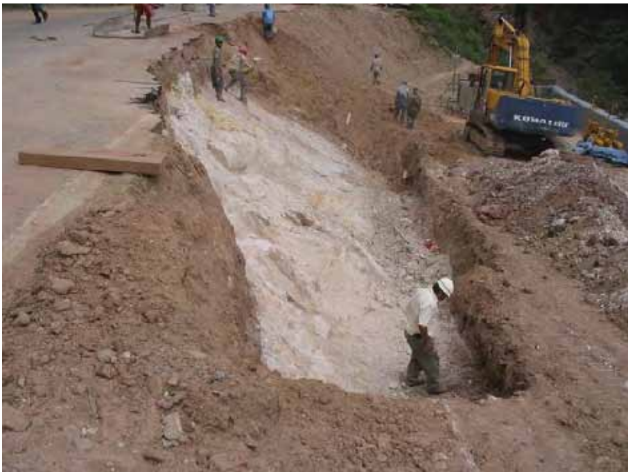
Photo 9.11.2 Reinforced soil wall bedrock (the bedrock crest is located approx. 2.0 m below the white line where the worker is standing.)
