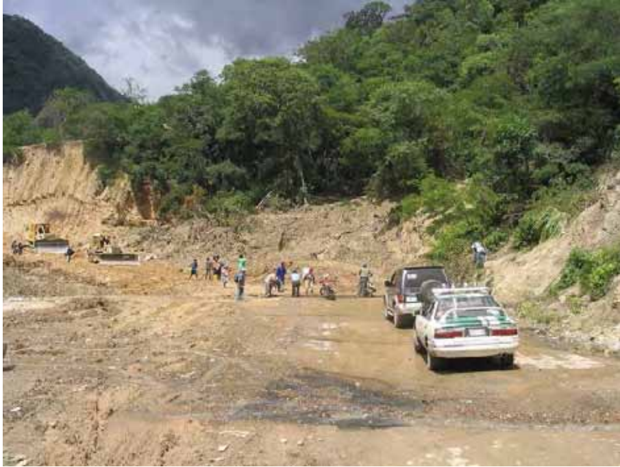
Photo 9.13.3 Collapsed road by debris flow (restoration work is under way)
