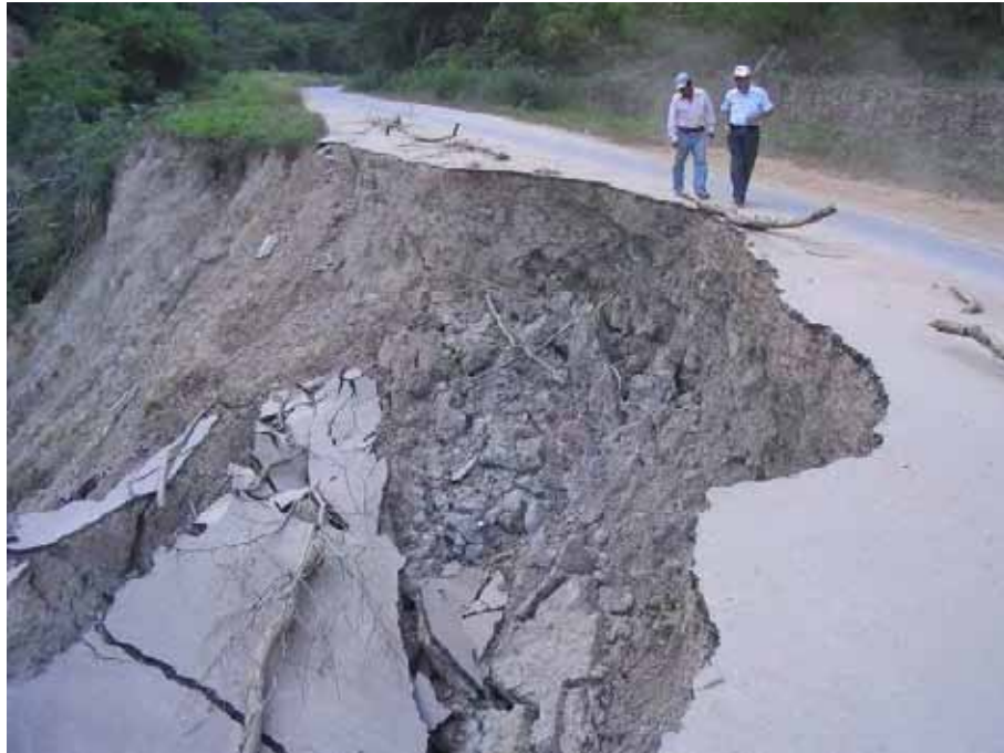
Photo 9.13.1 Collapse of road caused by rain water (1)
