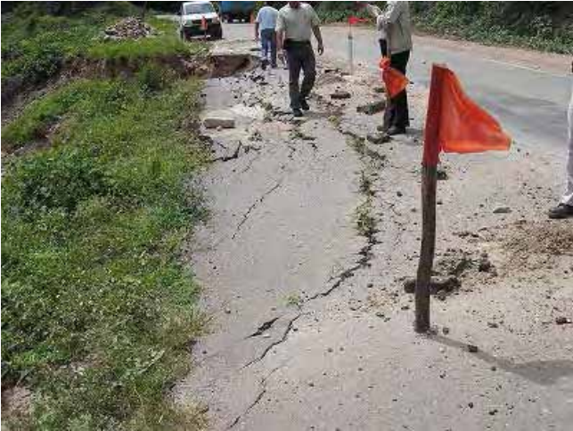
Photo 9.7.8 Open cracks in upper part of the landslide
