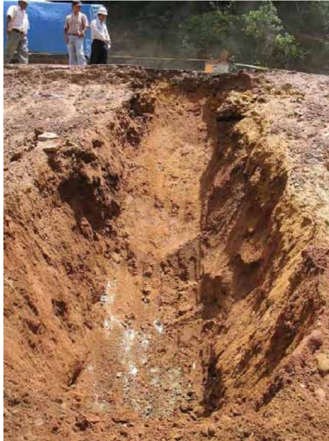
Photo 9.11.3 Unstable excavated surface due to poor construction work (Possible to excavate one power shovel operation)
