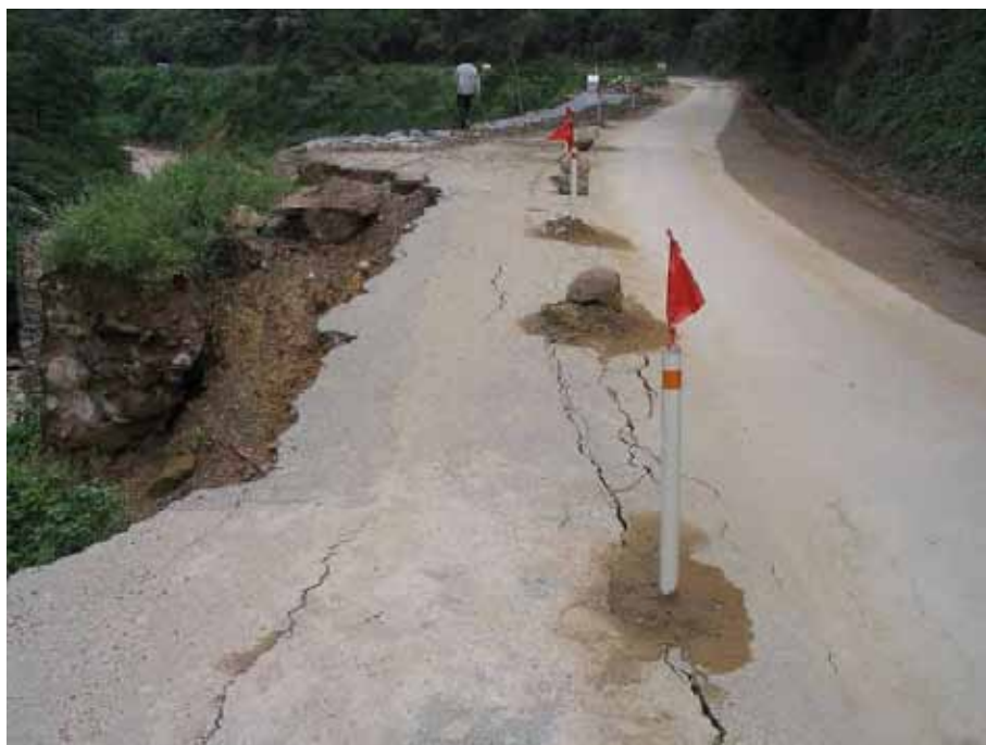
Photo 9.13.2 Collapse of road caused by rain water (2)
