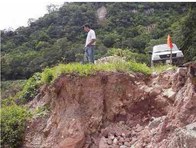
Photo 9.7.10 Secondary erosion by drainage water
