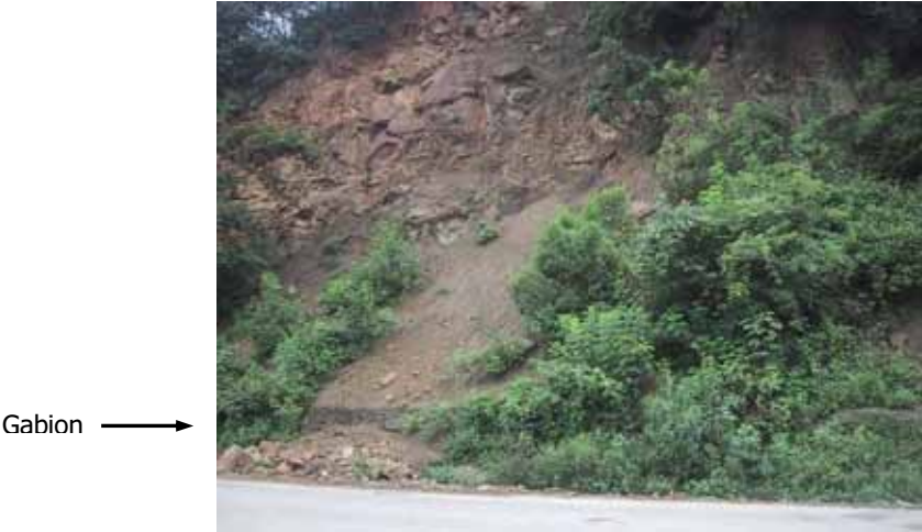
Photo 9.7.4 Gabion and piled rock-fall fragments
