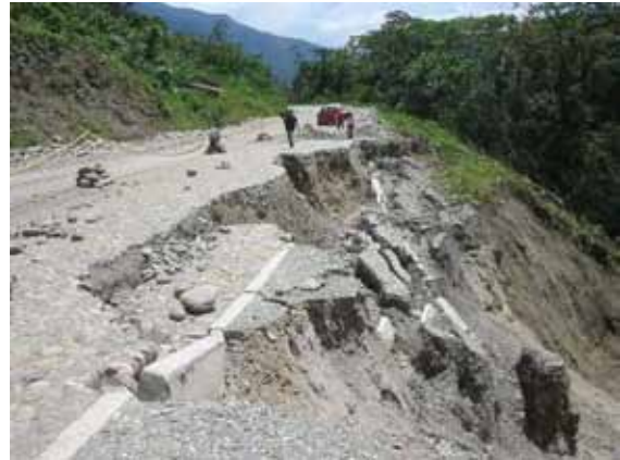
Typical slope failure at National highway No.4
